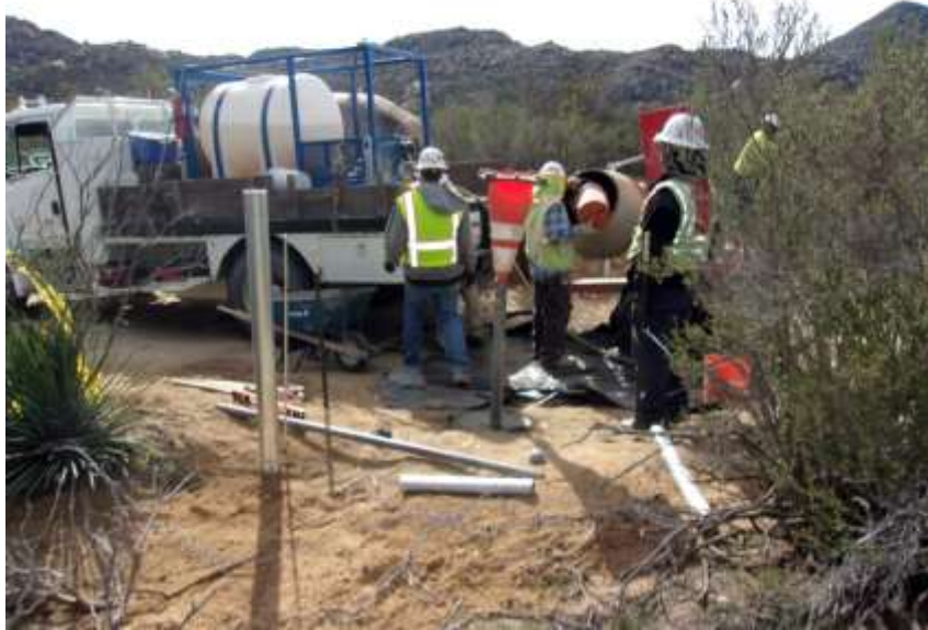
Photo 3: To minimize the potential for concrete spills on, sheets of Vizqueen were placed under the hand concrete mixer during fence installation along the overhead ROW. Fire watch was on site with fire tools in accordance with MM-FF-1.
