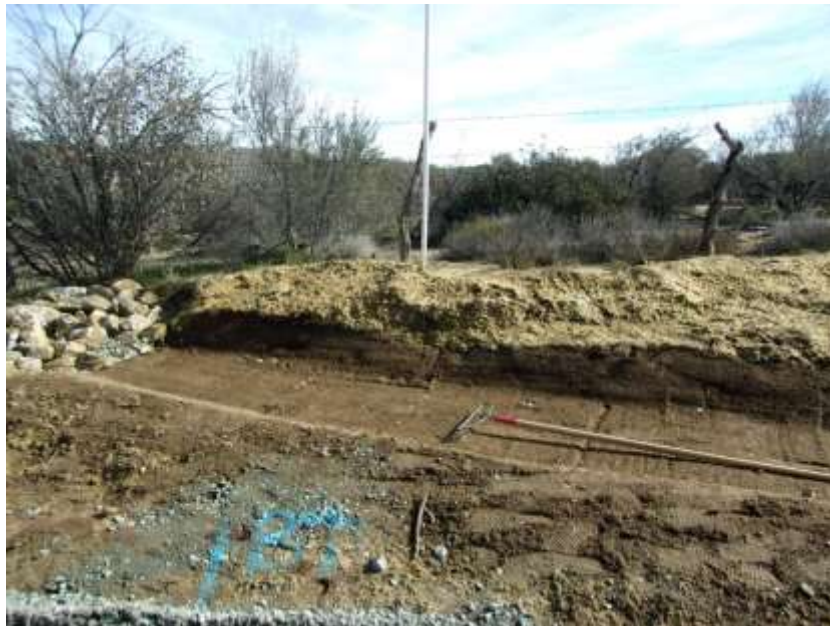
Photo 4: Rock drainages, water bars, and other erosion control devices along the ROW were completed and maintained according to the SWPPP and MM-HYD-1.
